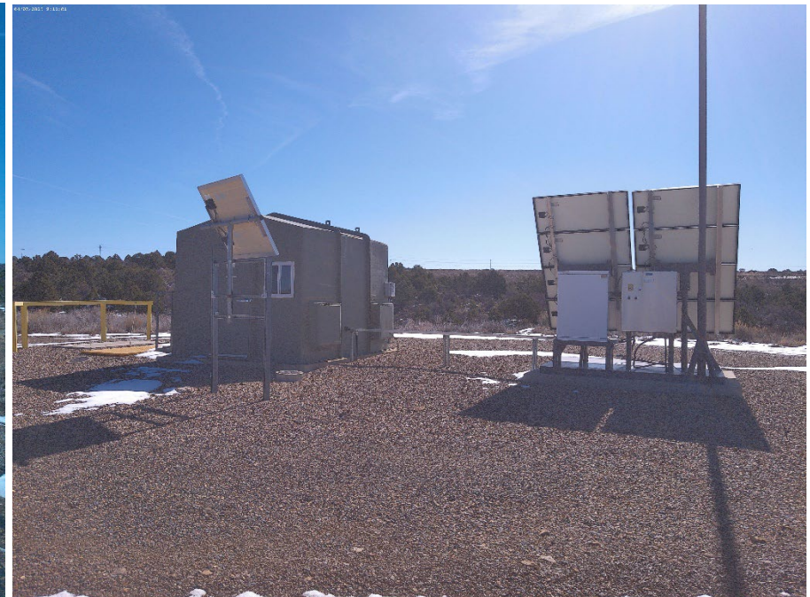
Injection Wellhead inside housing
