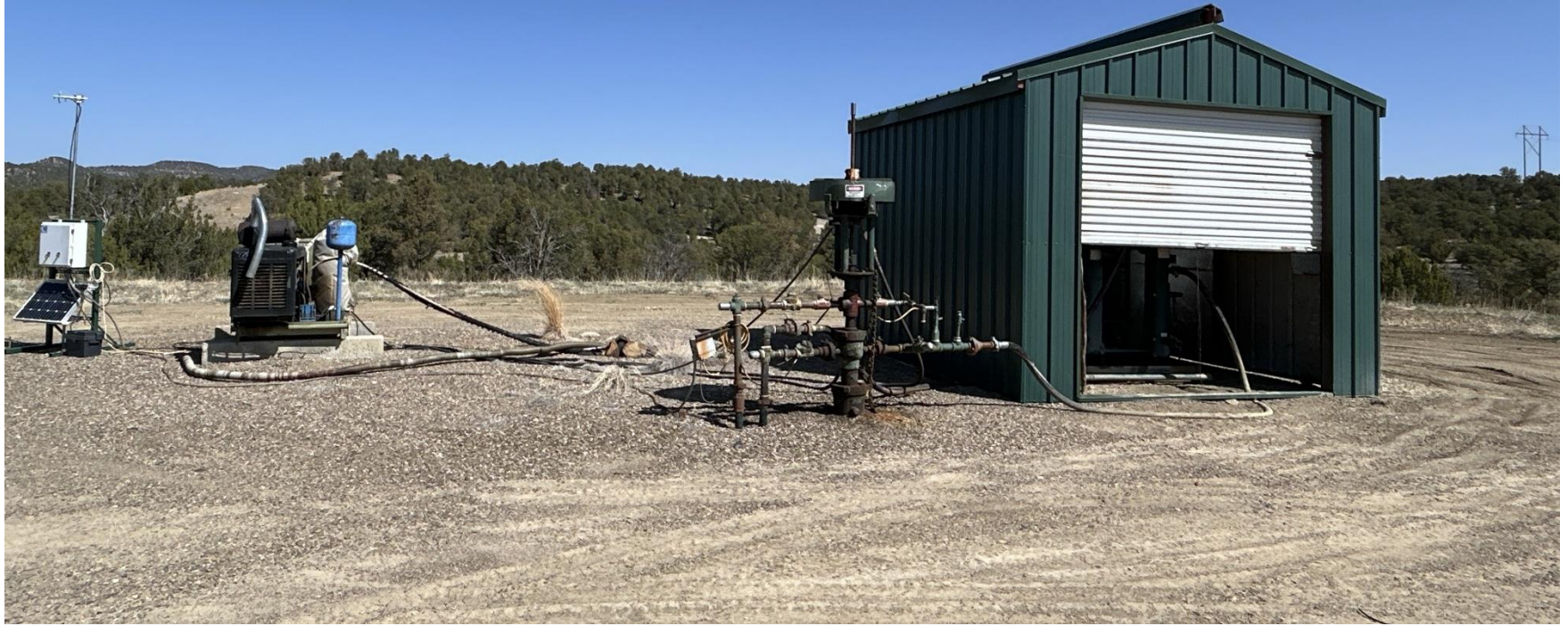
PHOTO 3: WELLHEAD AND EQUIPMENT
