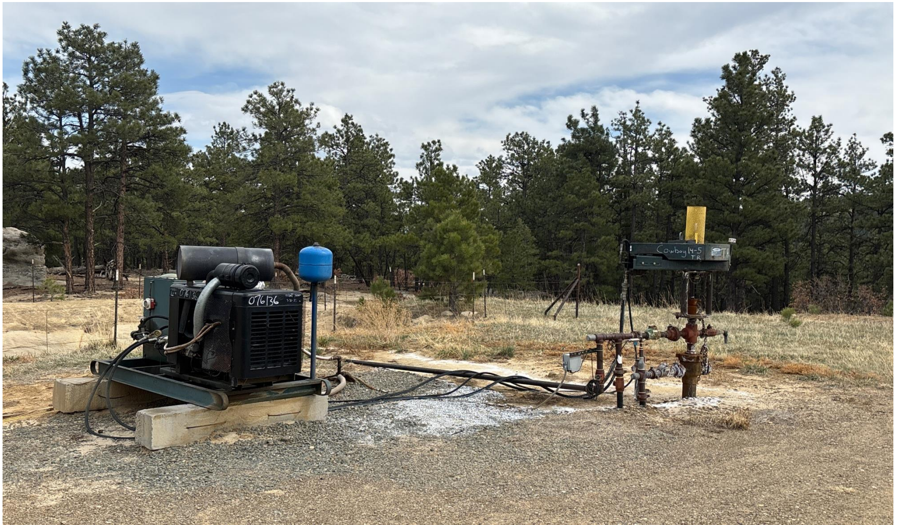
PHOTO 3: TR WELLHEAD AND EQUIPMENT.
