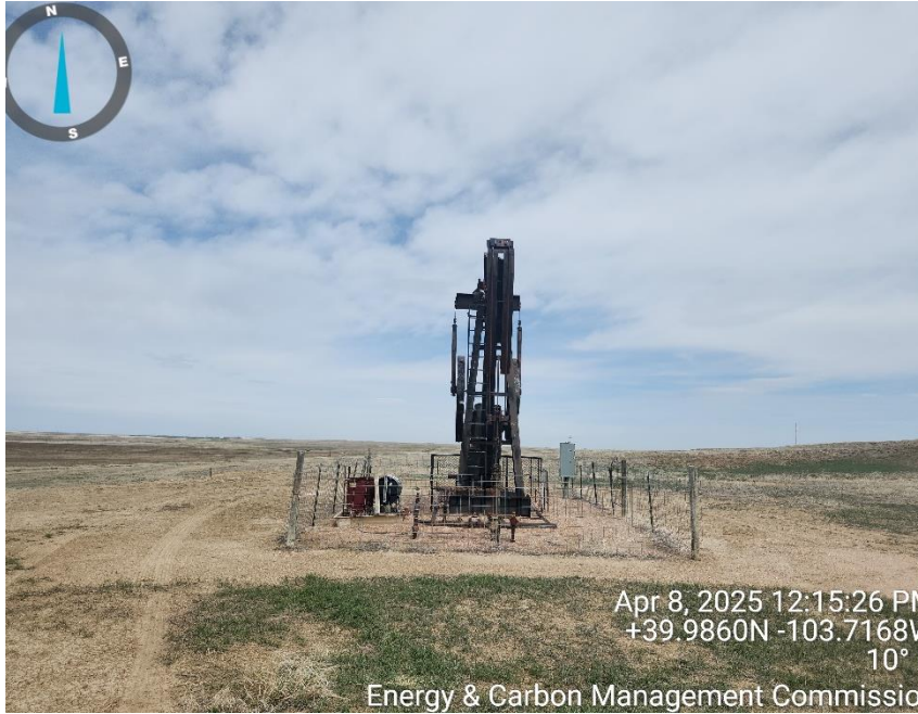
Photo 1 well head and equipment
