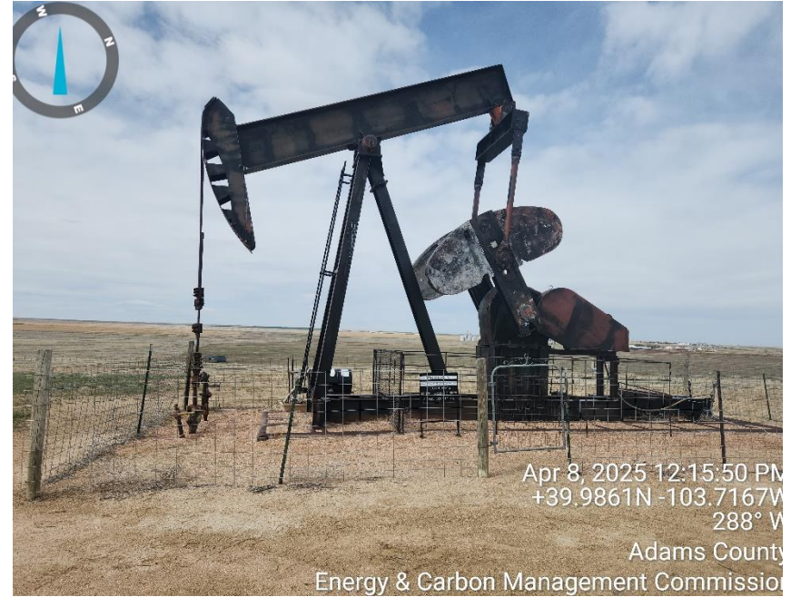
Photo 2 well head and equipment
