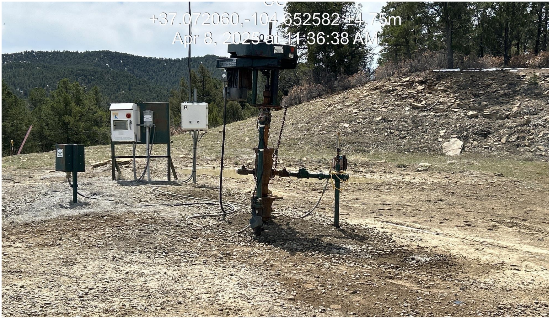
PHOTO 3: WELLHEAD AND EQUIPMENT
