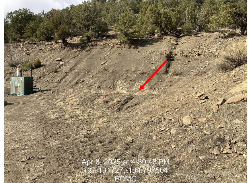
Photo 8 – BMP's full, Stormwater overtopping BMP's
