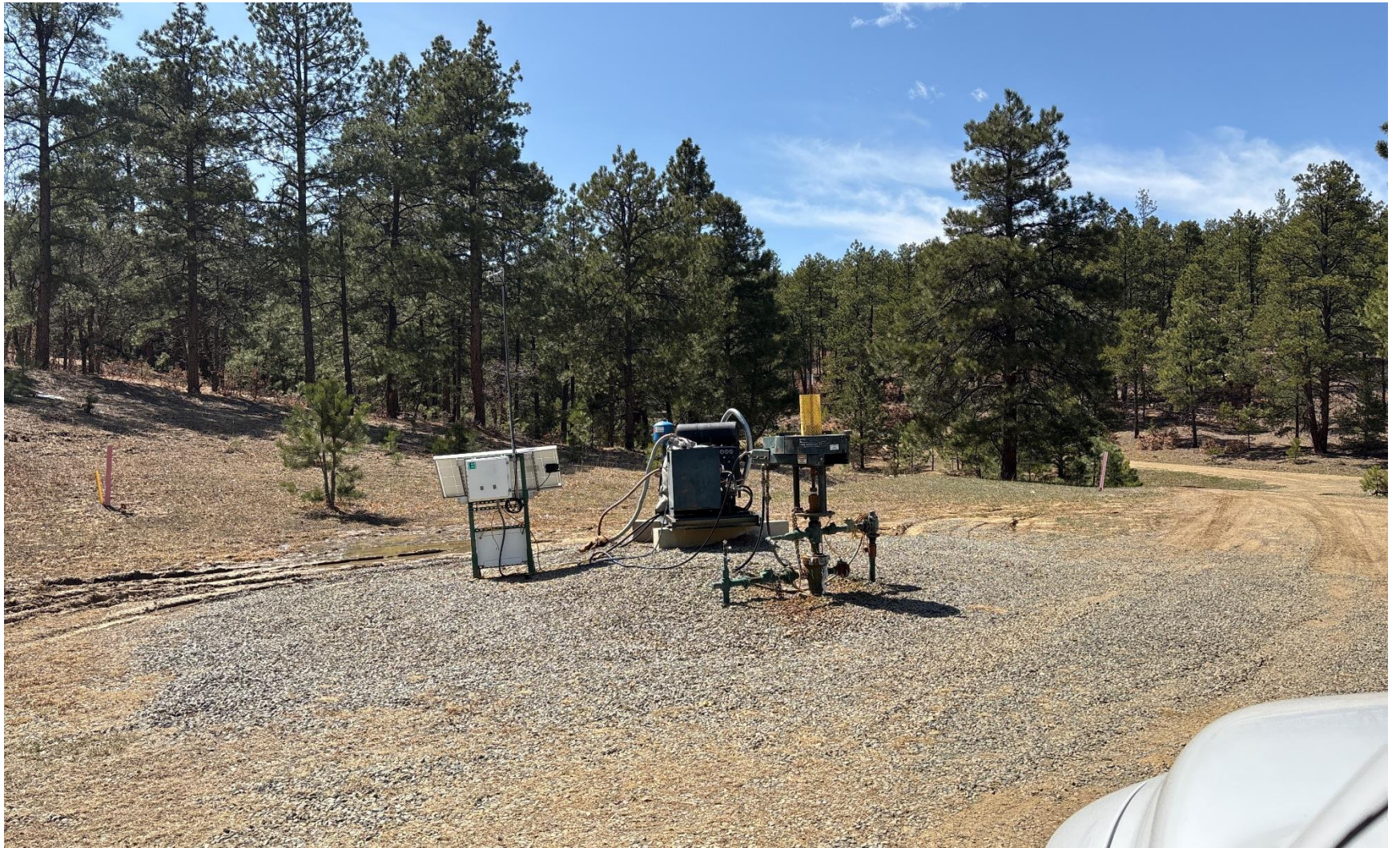
PHOTO 3: WELLHEAD AND EQUIPMENT.
