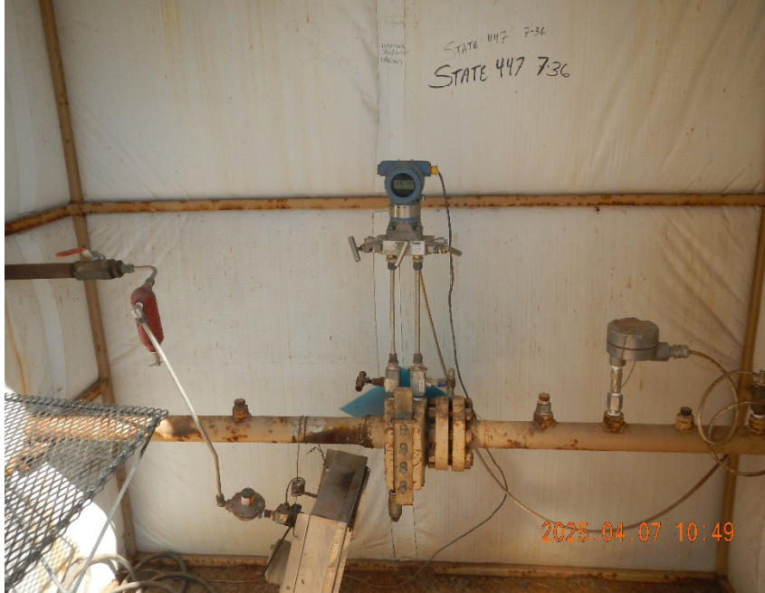
5. Gas meter inside meter shed.
