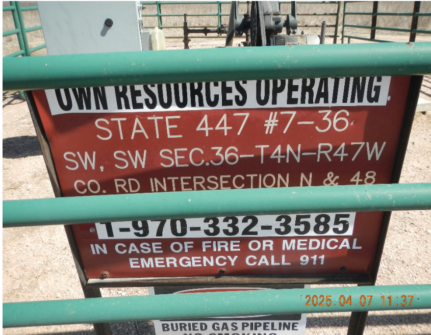
1. Lease sign at well location.
