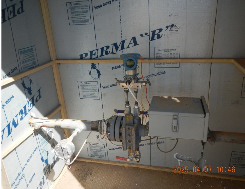
5. Gas meter inside meter shed.
