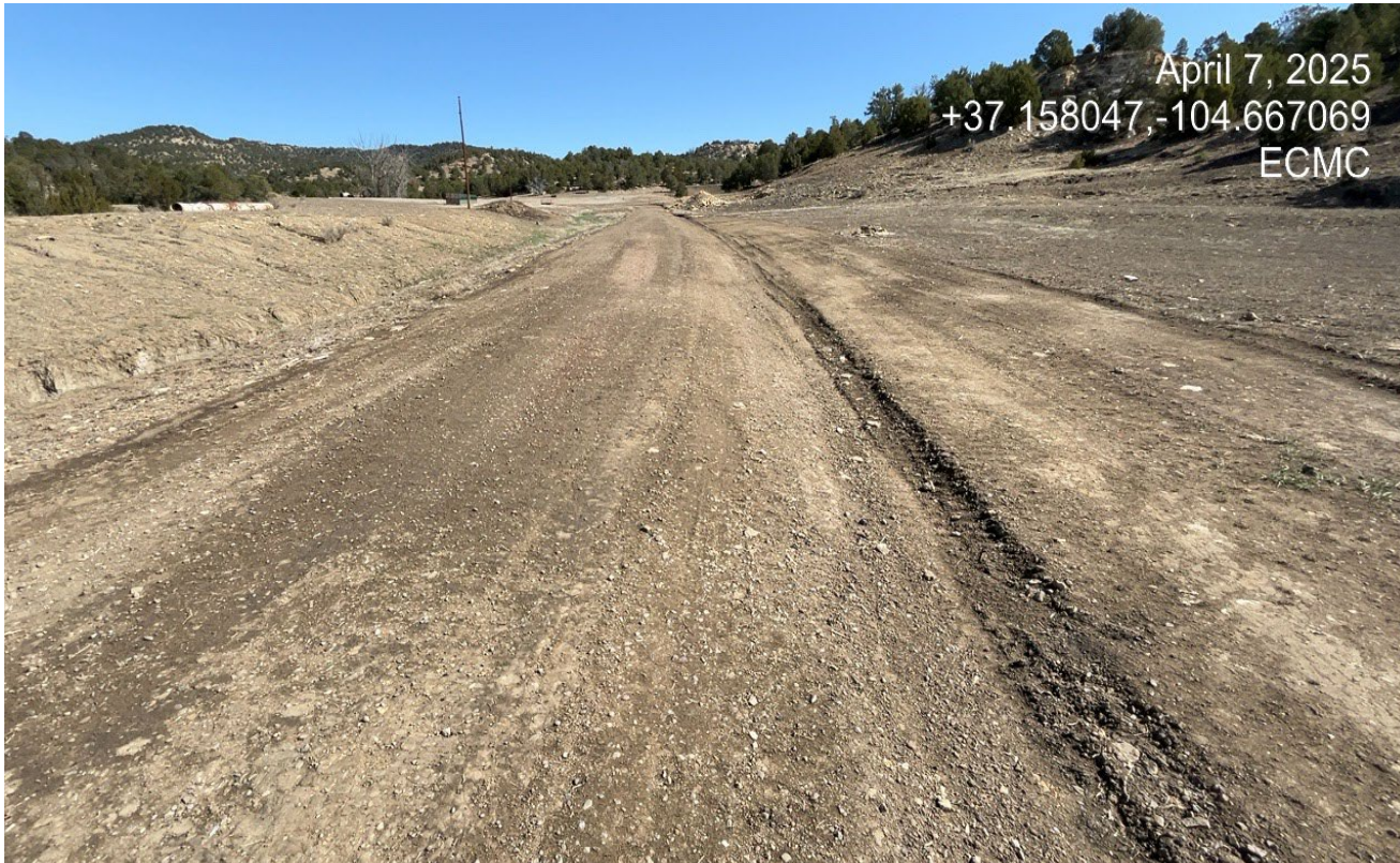
Photo 1. Facing northeast along the access road. This area of the road was repaired and seeded. This long stretch of road may require additional BMP's to prevent erosion until vegetation establishes.
