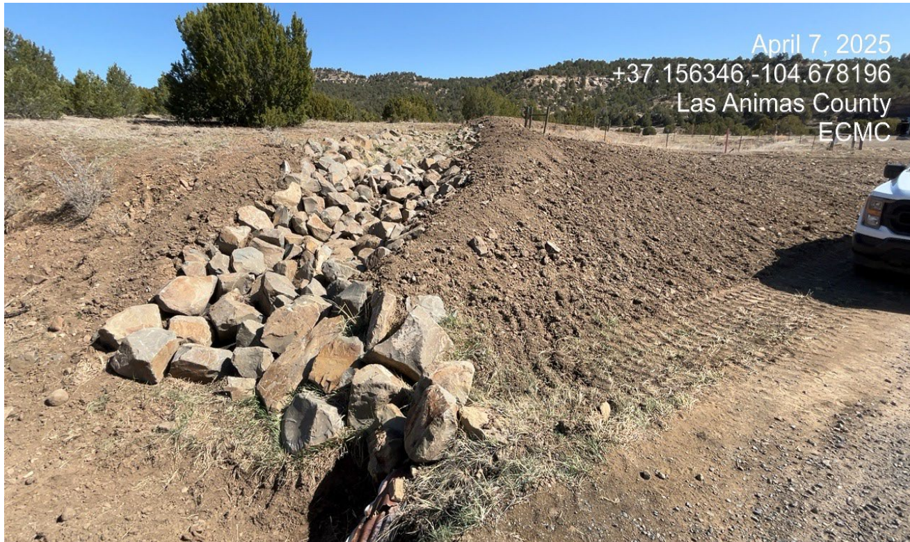
Photo 3. Facing toward the northwest side of the location. This area has been regraded and reseeded.
