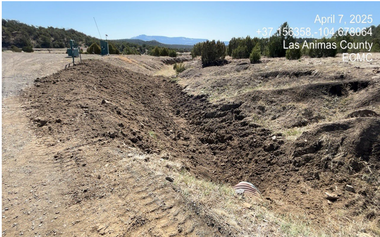
Photo 4. Facing southwest at the drainage crossing at the west side of the location. The culvert has been cleaned out and this area was reseeded..
