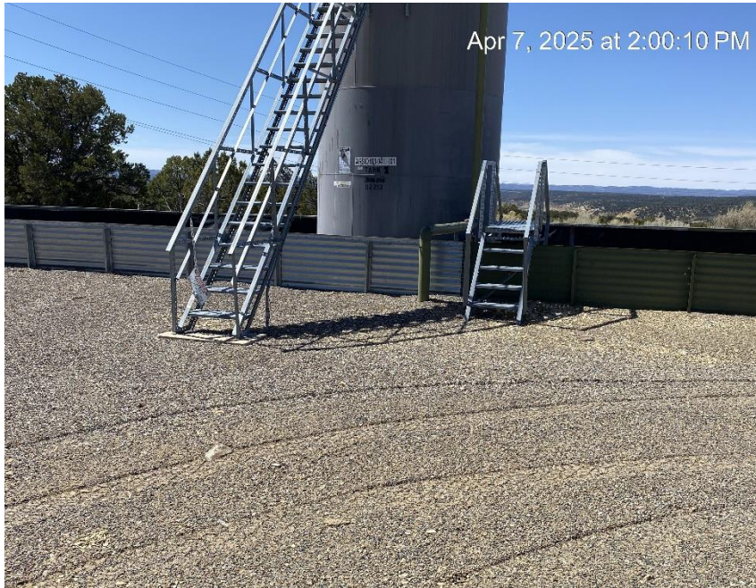
No tank battery sign
