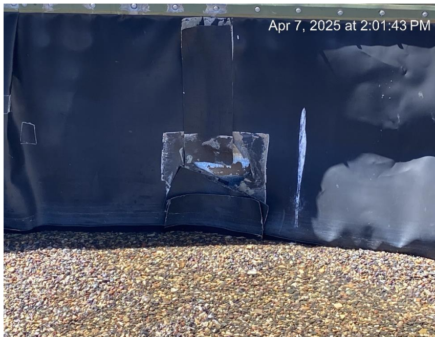
Insufficient liner repair
