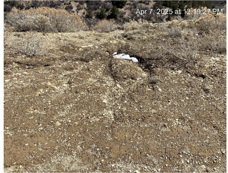
Stormwater BMP not maintained
