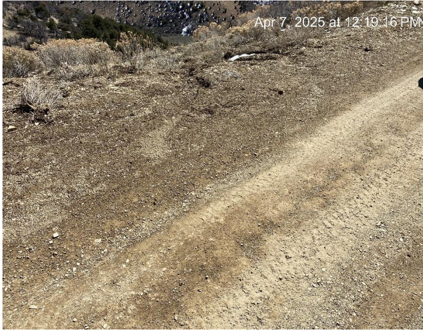
Erosion and sediment migration
