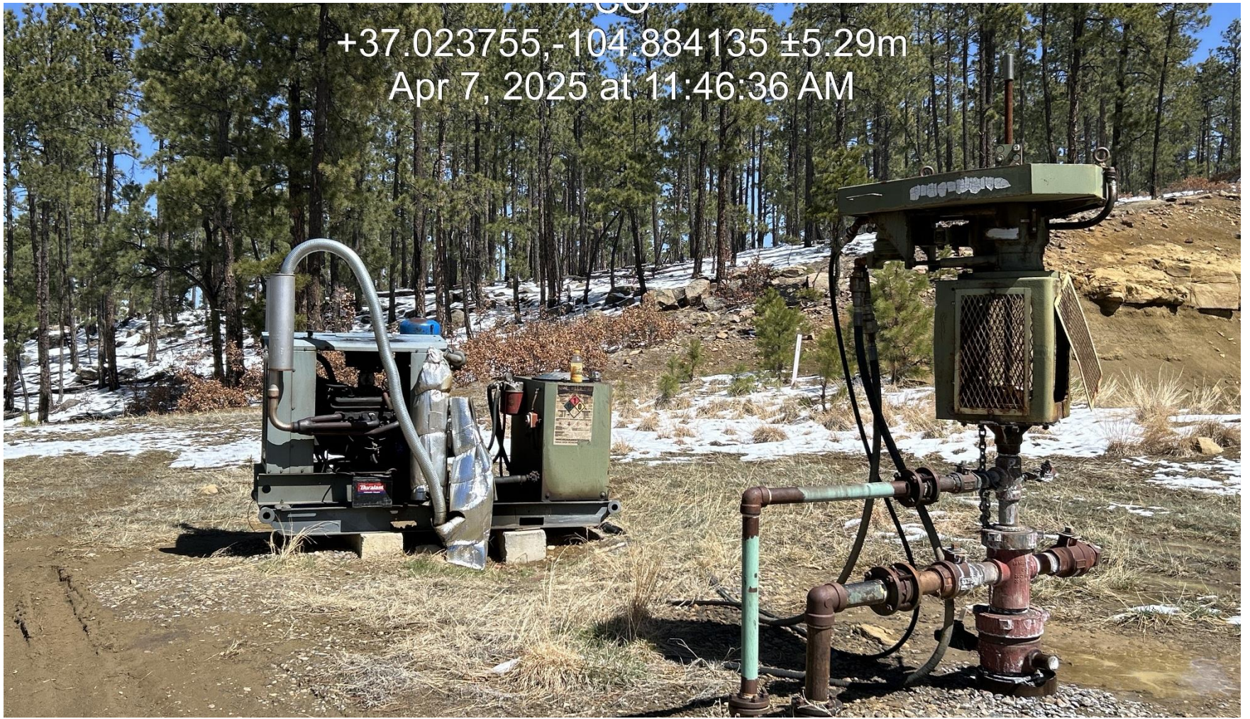
PHOTO 3: WELLHEAD AND EQUIPMENT
