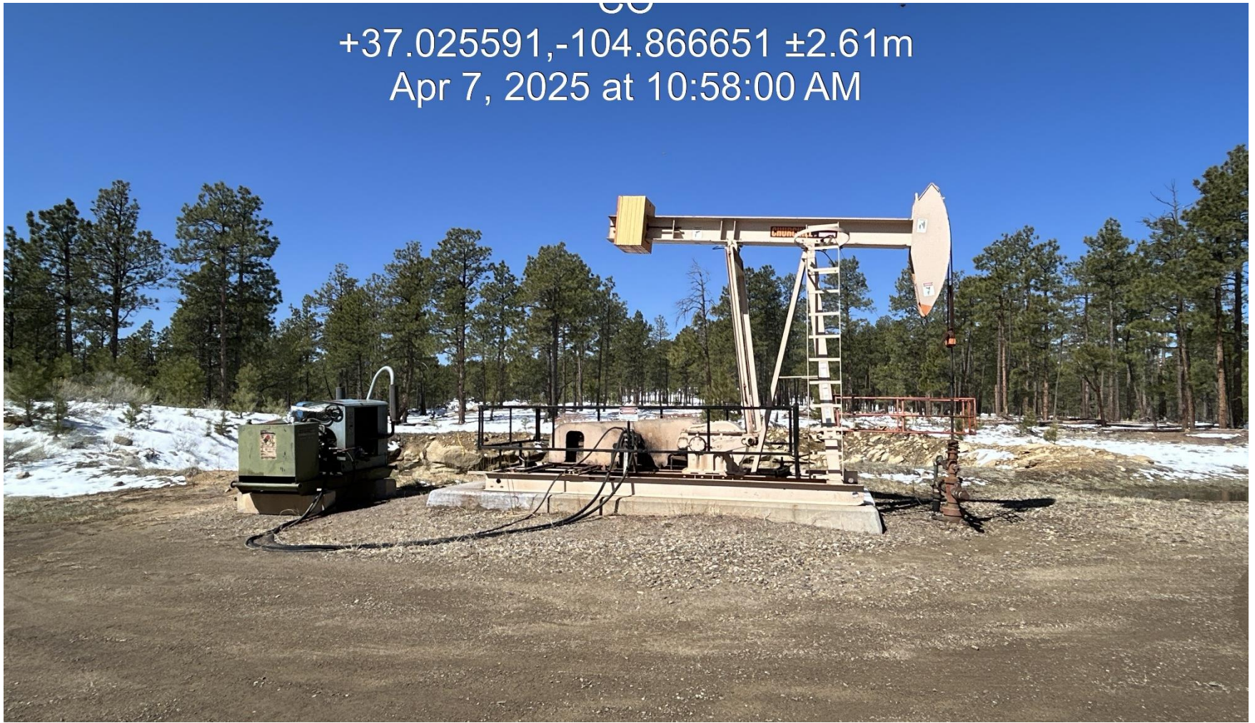
PHOTO 3: WELLHEAD AND EQUIPMENT
