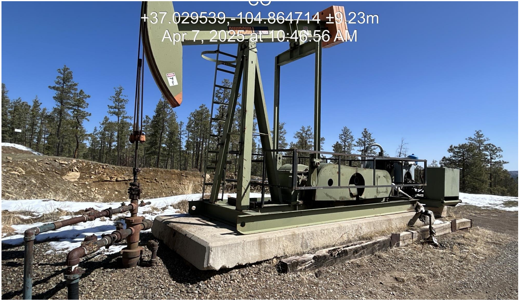
PHOTO 3: WELLHEAD AND EQUIPMENT
