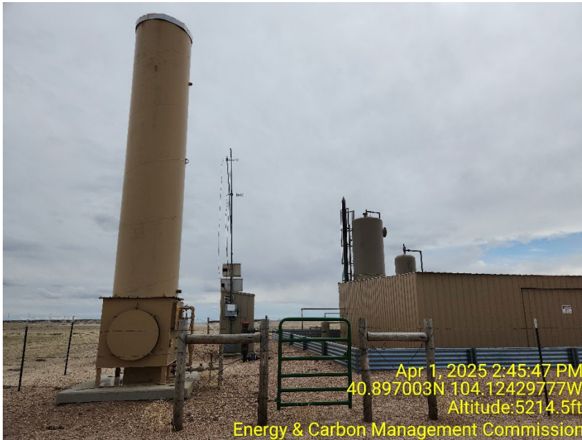
Photo 1 – ECD and Heater Treater
