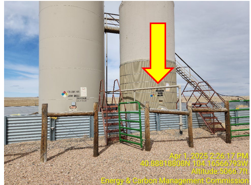
Photo 8 – Tank Battery – NFPA on Water Tank
