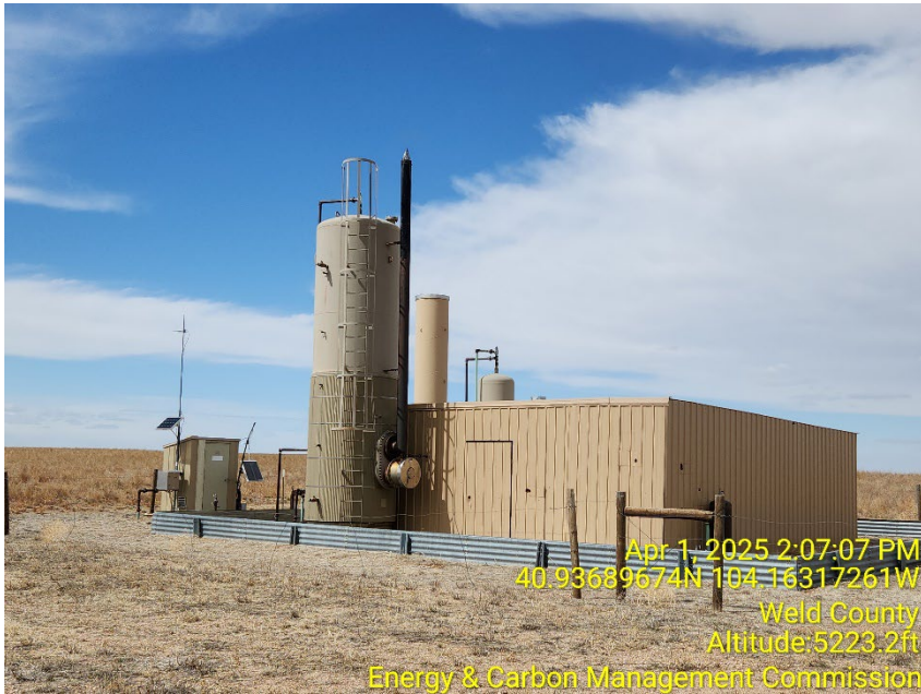
Photo 5 – Heater Treater and ECD
