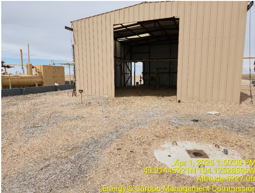
Photo 5 – Sign need reinstalled at Vault
