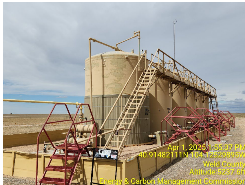
Photo 8 – Tank Battery – Sign missing
