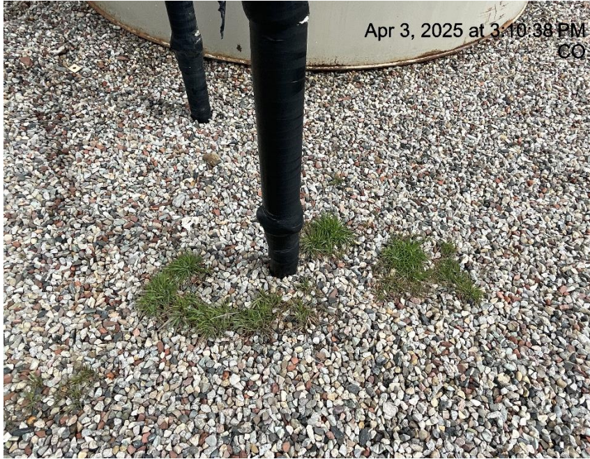
Photo # 9060 Weeds in secondary containment
