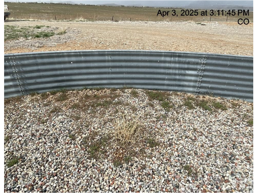
Photo # 9061 Weeds in secondary containment
