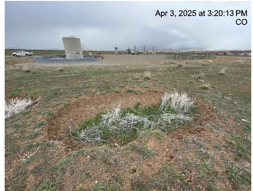
Photo # 9063 Subsidence in the interim area
