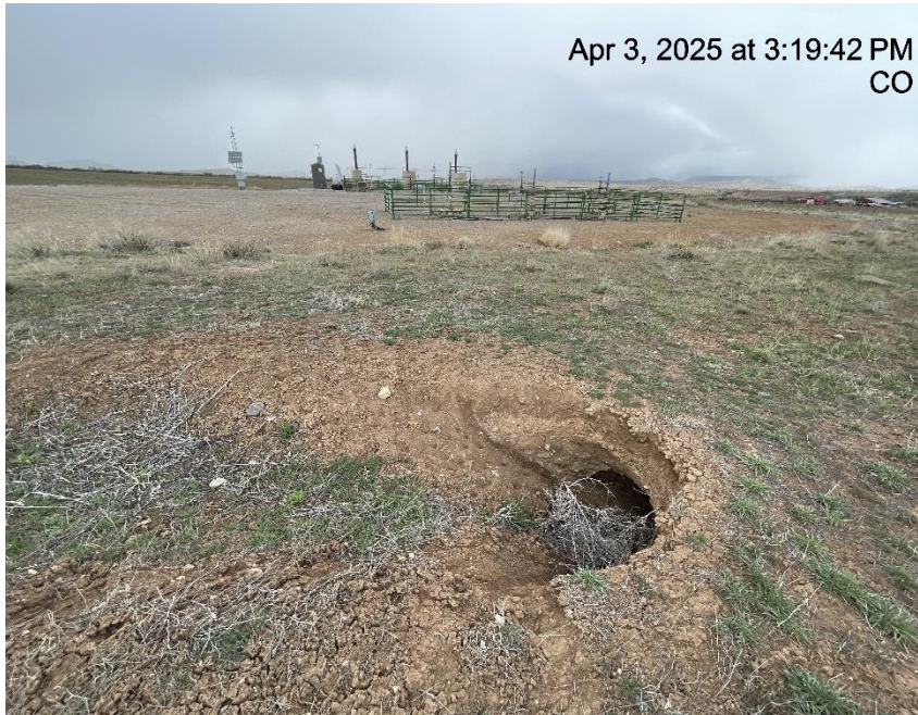
Photo # 9062 Subsidence in the interim area
