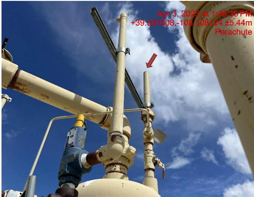
Photo # 6918 Rupture disc vent line does not comply with CECMC pressure safety device rules
