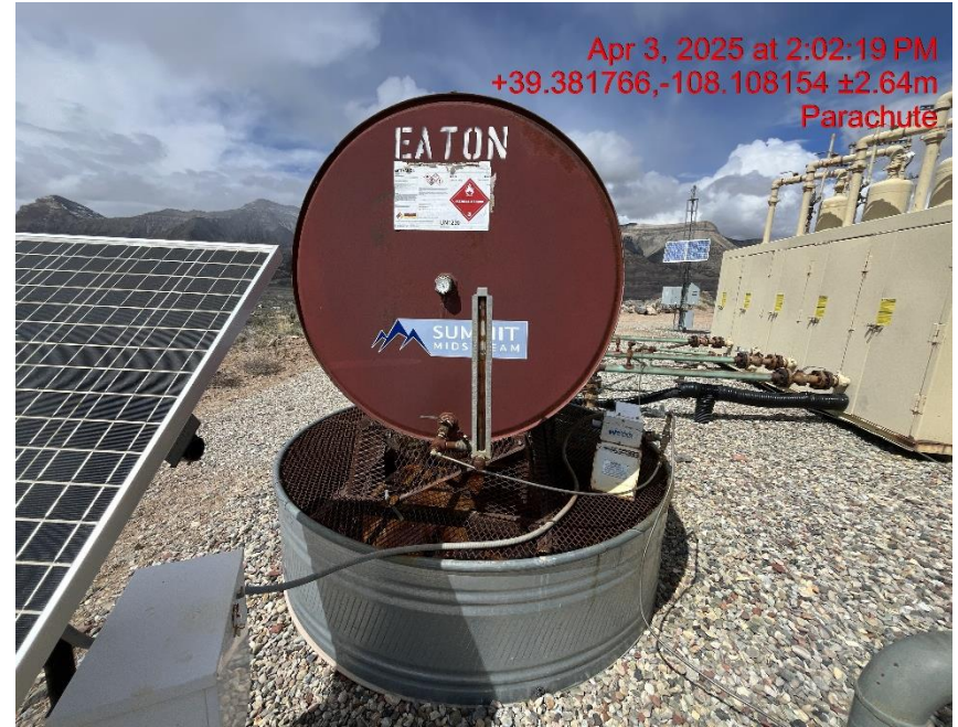
Photo # 6932 Methanol tank lacks required labeling/does not comply with CECMC rules
