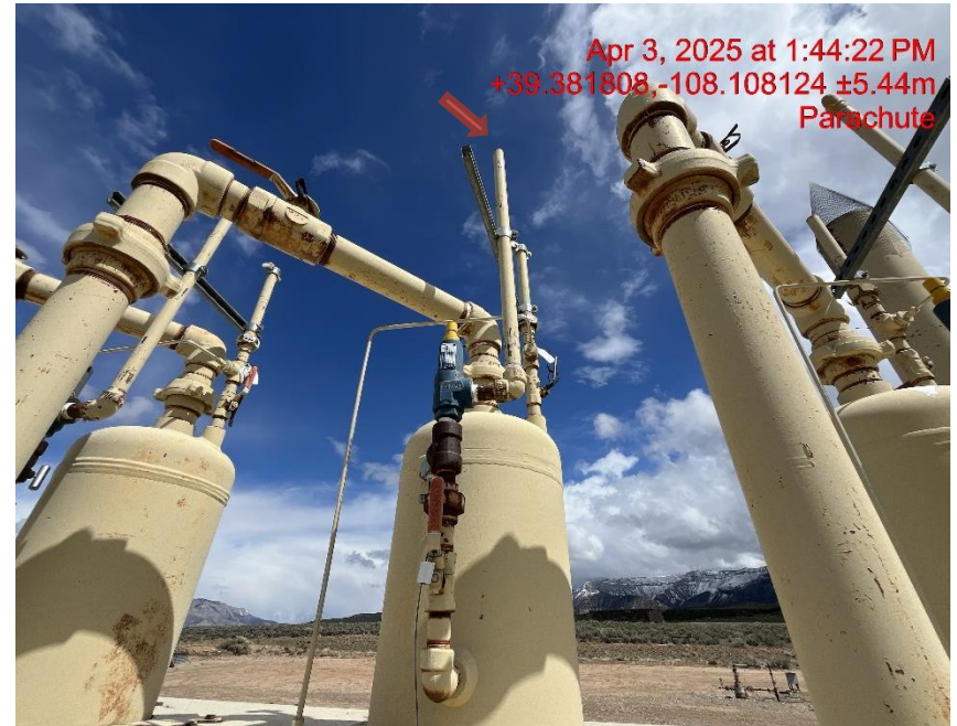
Photo # 6914 PRV vent line does not comply with CECMC pressure safety device rules
