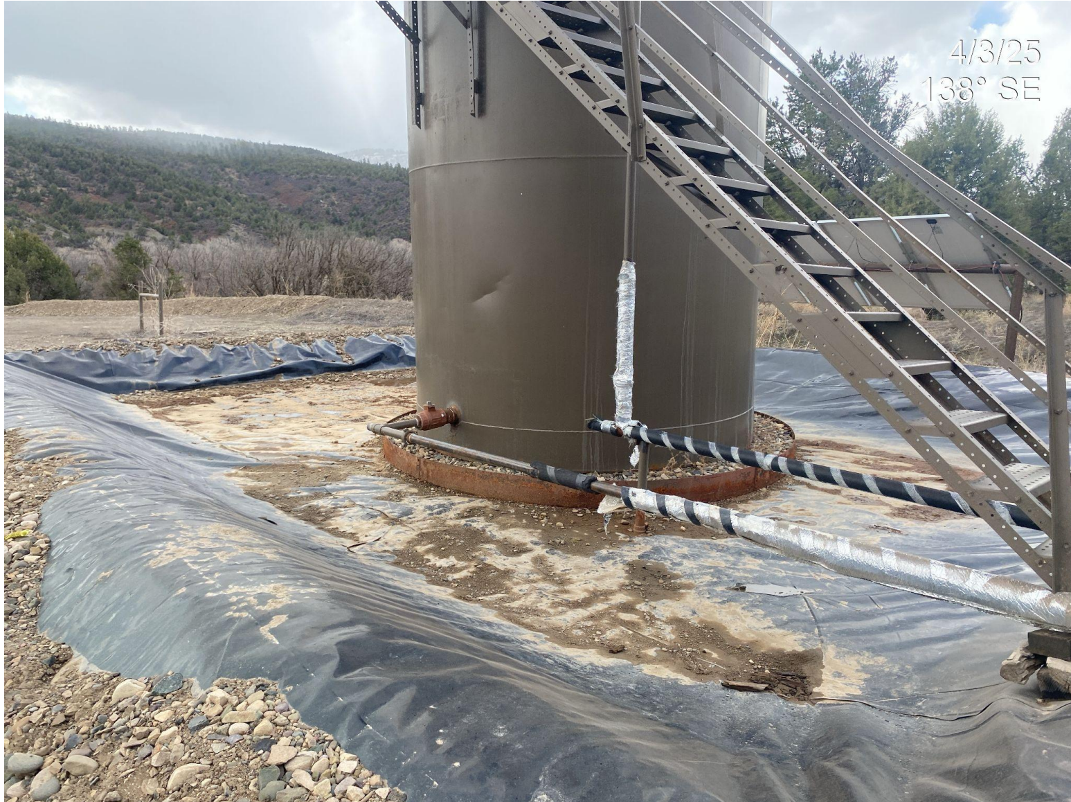
Photo 2. Gravel has been removed from produced water tank secondary containment.
