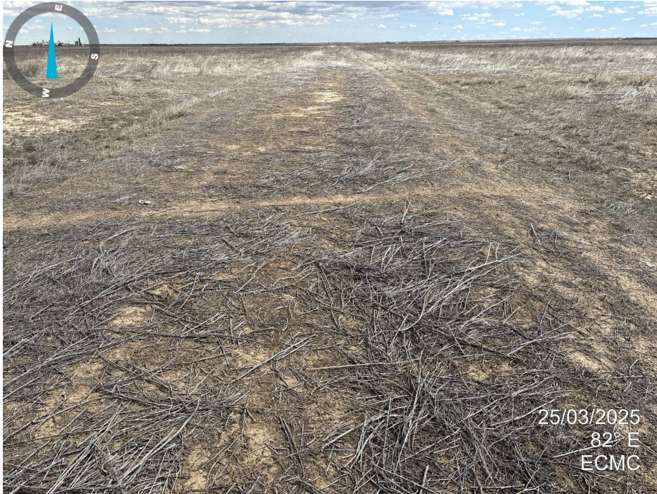
Photo 3. Looking east down access road near fence line. Very little desirable vegetation establishment on access road, especially towards the west side. The crown of the road is visible in this picture, the road is elevated above the surrounding area and ditches are present on both sides.
