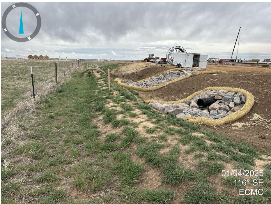
Photo 15. Looking east down the north side of location. Outlets are reinforced and a sediment trap is present.
