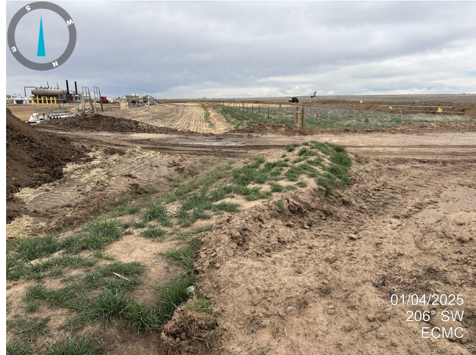
Photo 14. Looking south down the west side of the location. The ditch and berm have been removed. It does not appear that the ditch can convey water to the sediment trap.
