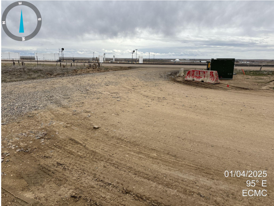
Photo 3. Riprap behind track out pad is full of sediment
