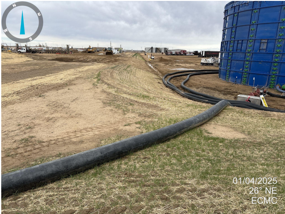
Photo 9. Looking north between the pad and production facilities. Slope appears to have been stabilized and seeded with evidence of germination.
