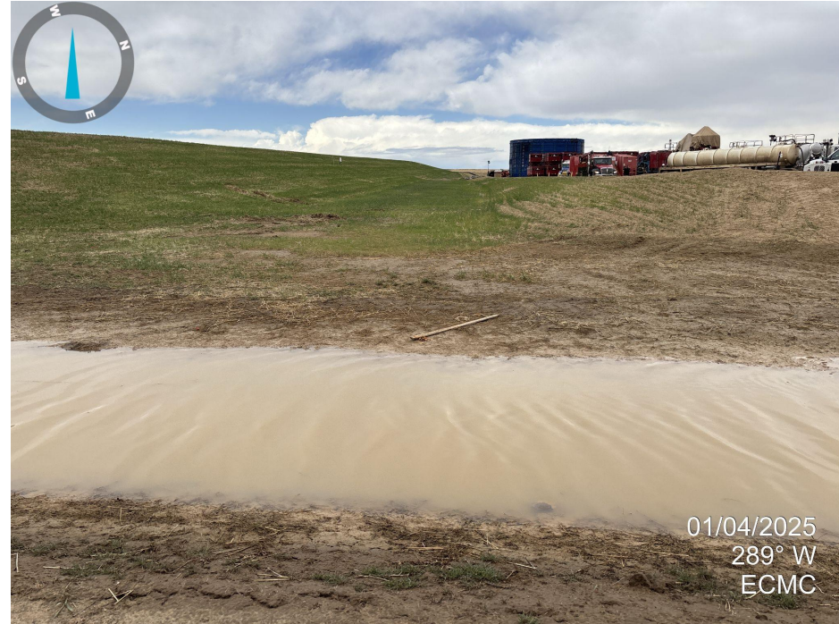
Photo 6. Looking west between the southern topsoil stockpile and pad. Area appears stabilized with vegetation germination.
