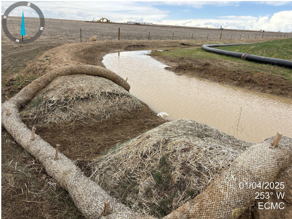
Photo 7. Picture taken at sediment trap at southwest corner of location. It does not appear that sediment is leaving the location.
