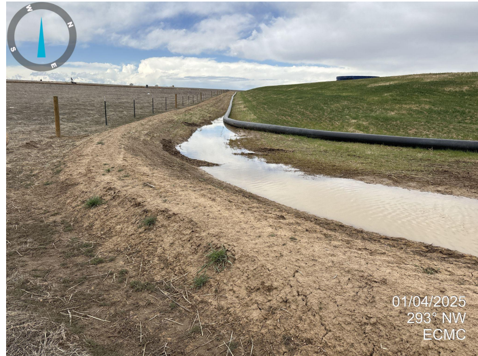
Photo 8. Looking west along the southern edge of location. Southern topsoil stockpile appears to be stabilized with germination of vegetation.
