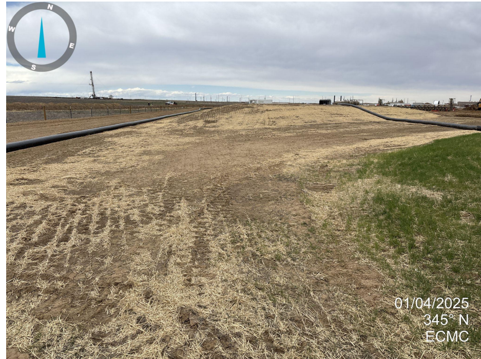
Photo 10. Triangular shaped topsoil stockpile on the west side of location. Stockpile appears to have been stabilized with crimped straw.
