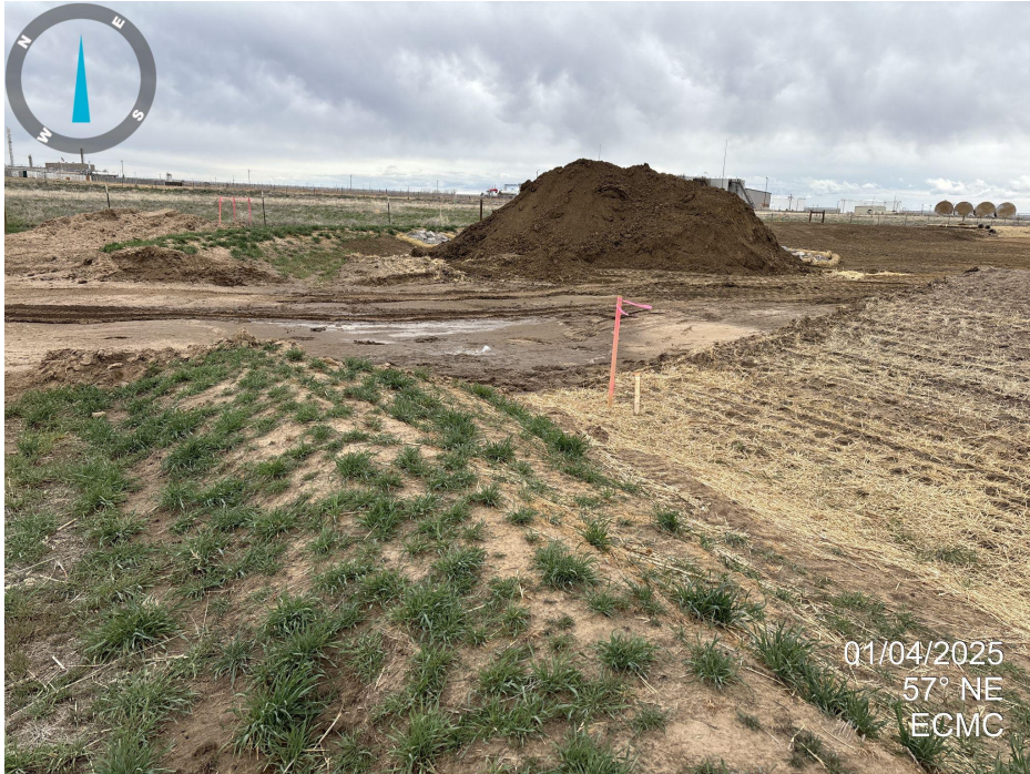
Photo 13. Looking northeast down the west side of the location. The ditch and berm have been removed for access out the west side of location. A culvert is not present and the road is muddy over the ditch. A soil pile without erosion BMPs is present.
