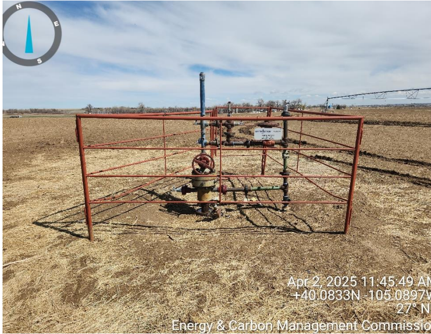
Photo 1 well head and equipment
