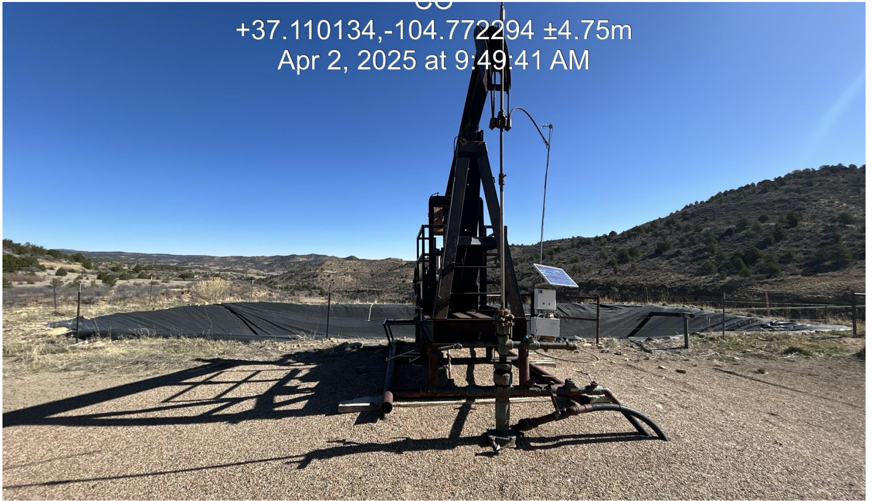
PHOTO 3: WELLHEAD AND EQUIPMENT
