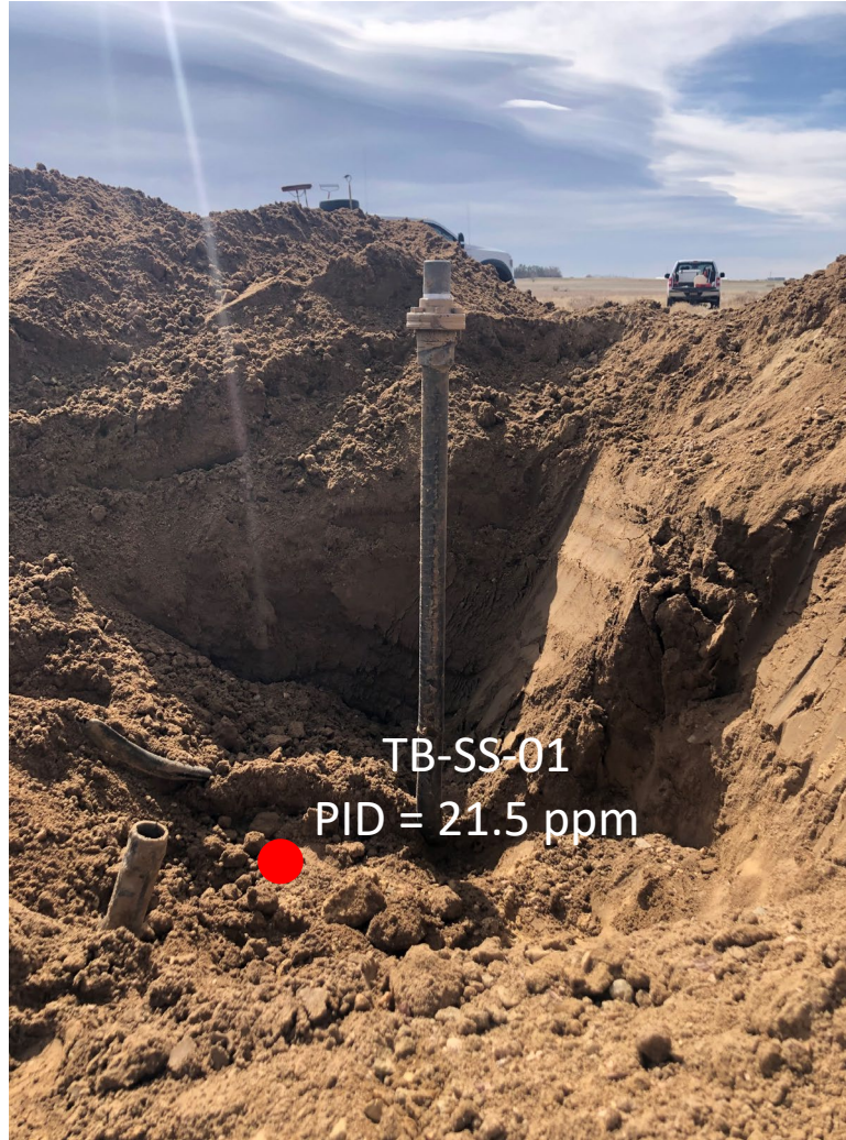
Looking south at flowline from wellhead
