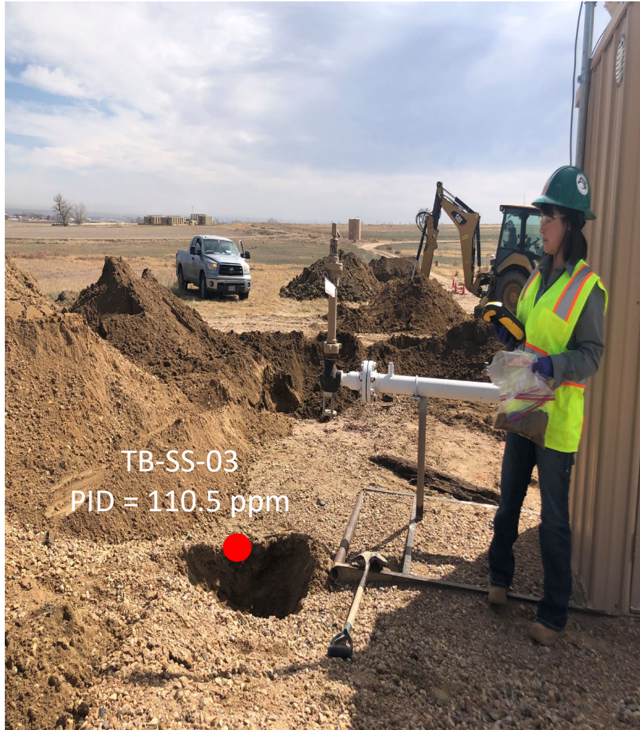
Looking east at meter house screening sample
