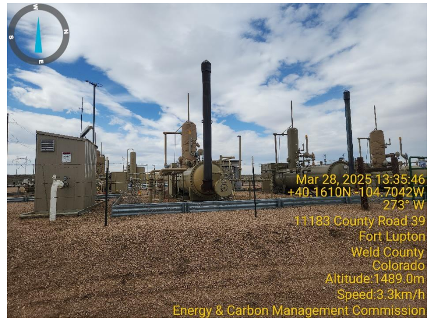
Photo 2 Horizontal Heated Separators.
