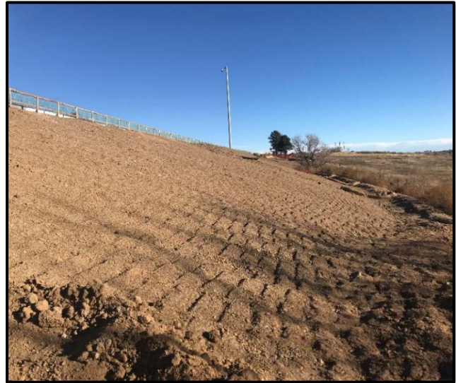
Vertical tracking on disturbed side slope
