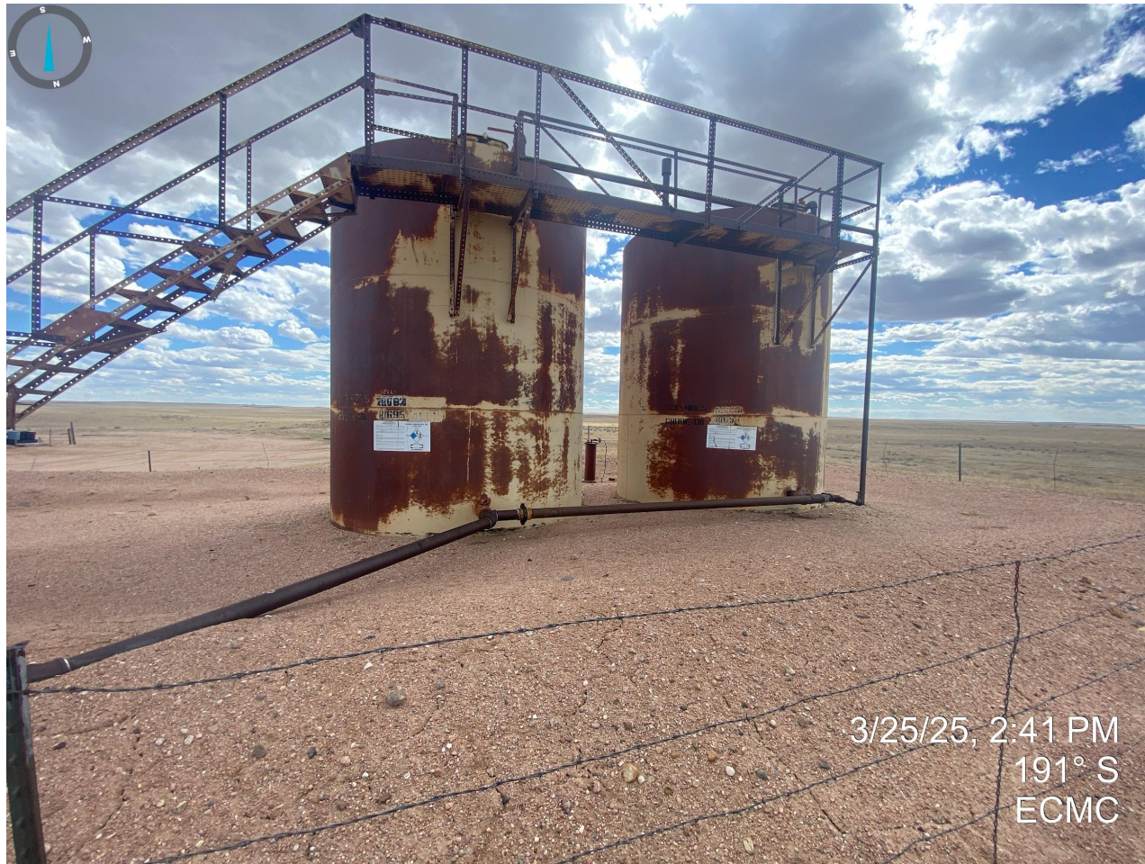
Photo 3. Tank labels/placards are faded/peeling/cracked and require replacement.
