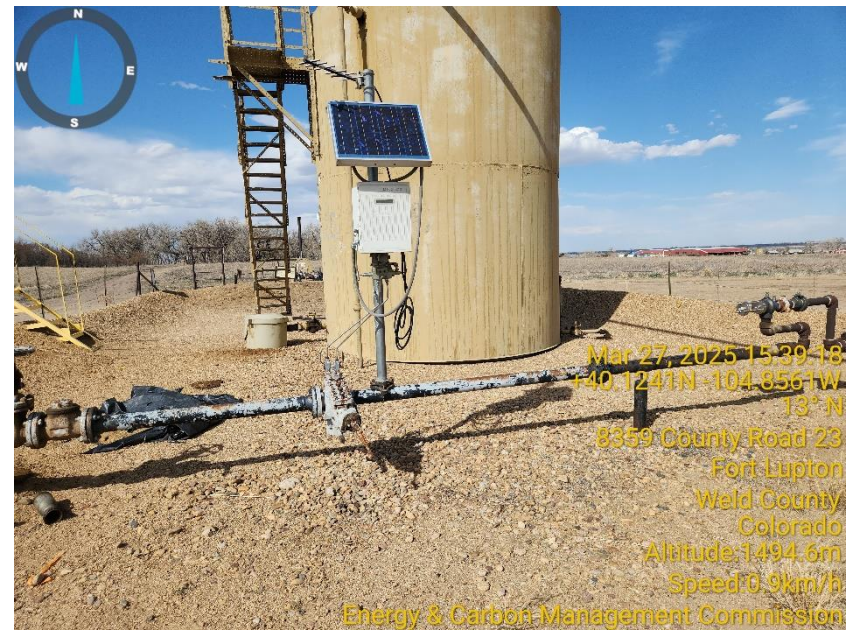
Photo 8 Gas Meter run.
