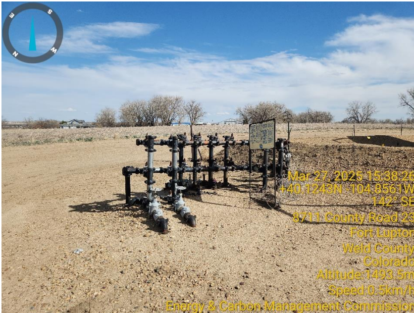
Photo 7 Flow line manifold.
