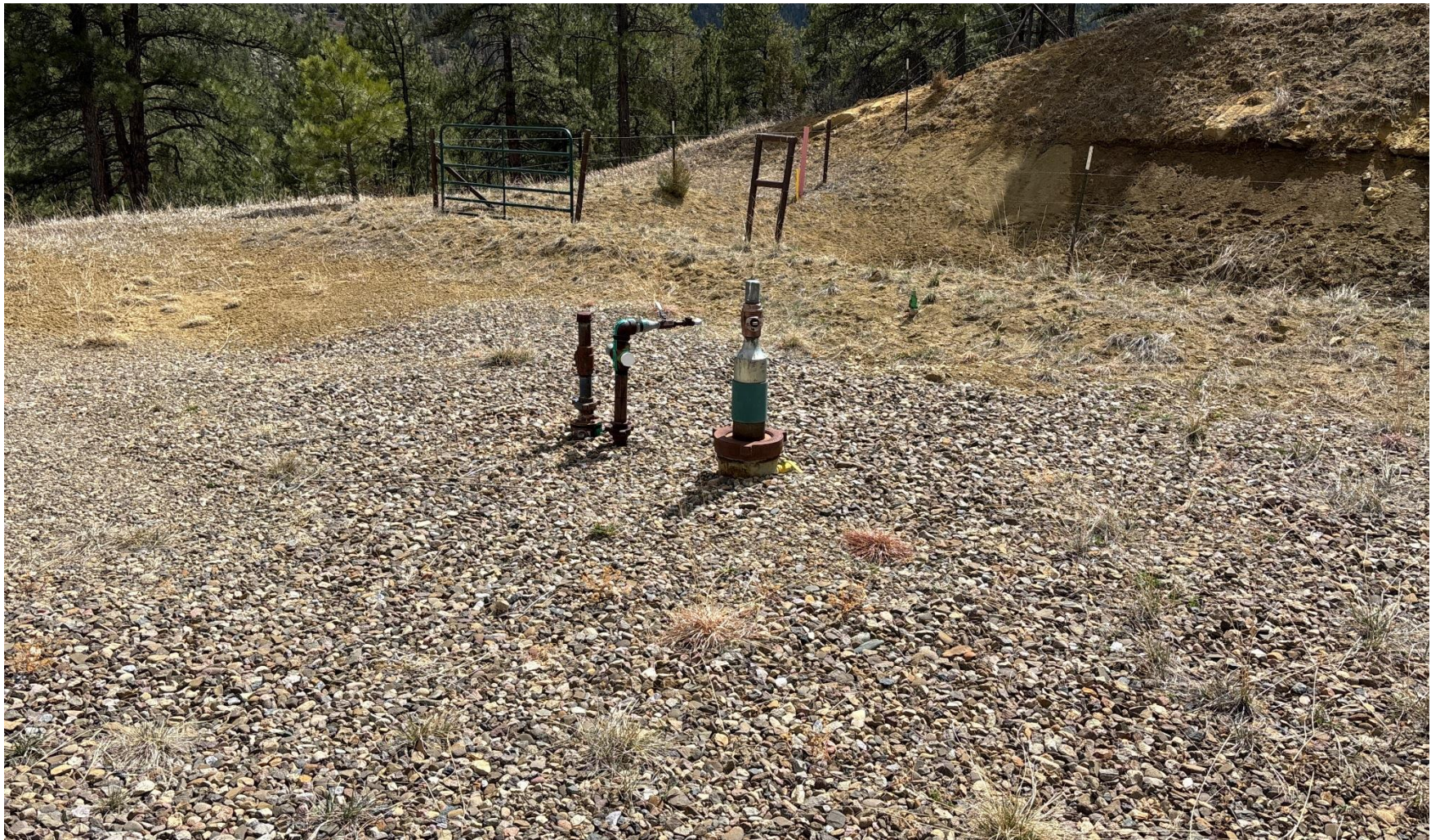
PHOTO 4: TR WELLHEAD AND EQUIPMENT./ WELLS NEED TO BE IDENTIFIED AT WELLHEAD.
