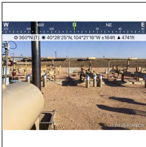
P1 - Looking north from the center of the Site excavation. The facility has returned to production following the excavation.
