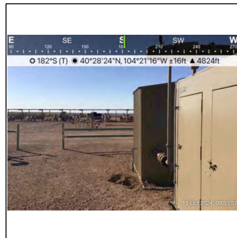
P3 - Looking south from the center of the Site excavation. The facility has returned to production following the excavation.
