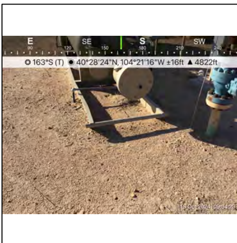
P5 - Excavation area up close, clean backfill and road base has been emplaced to match the existing Site contour.
