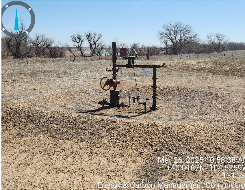
Photo 1 well head and equipment
