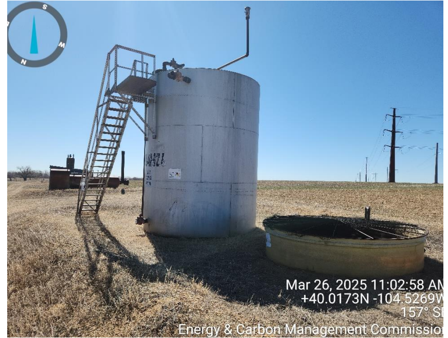
Photo 4 production equipment & tank battery
