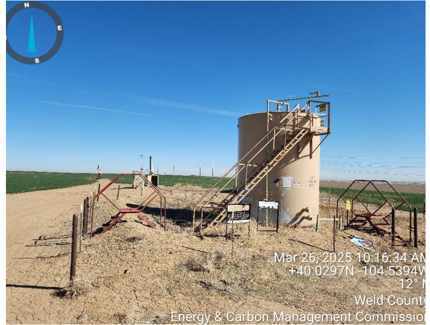
Photo 2 production equipment and tank battery
