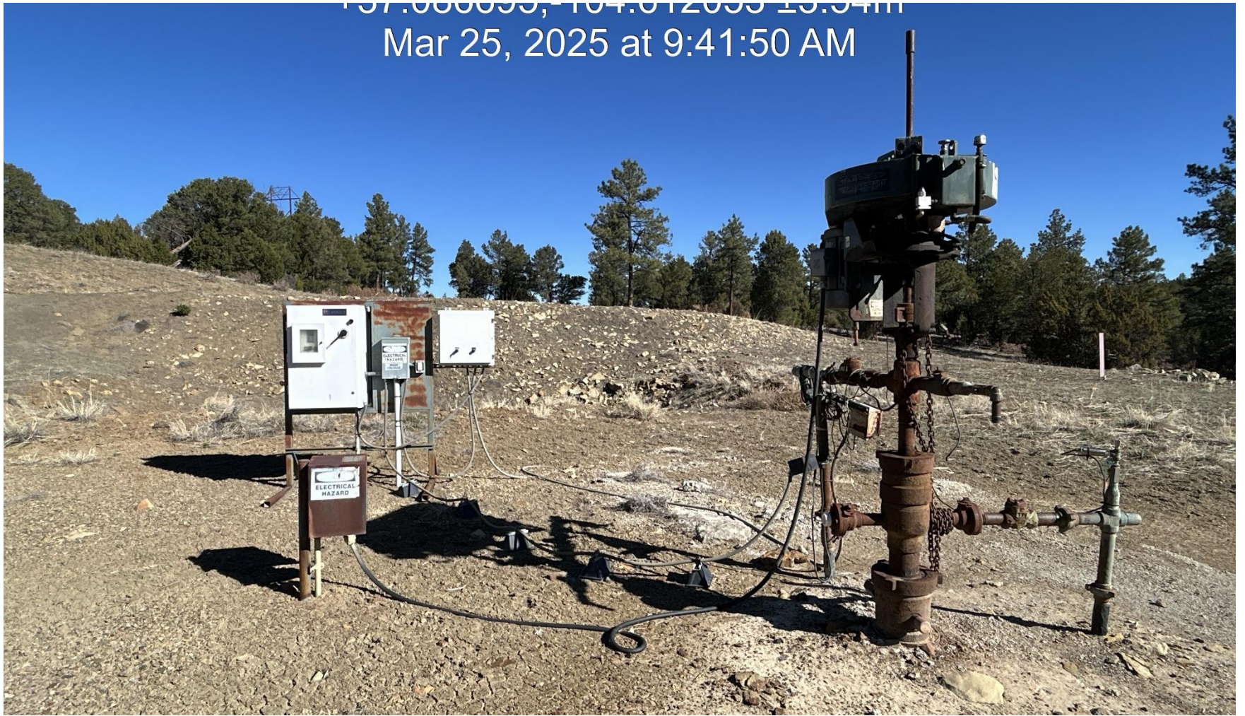
PHOTO 3: WELLHEAD AND EQUIPMENT
