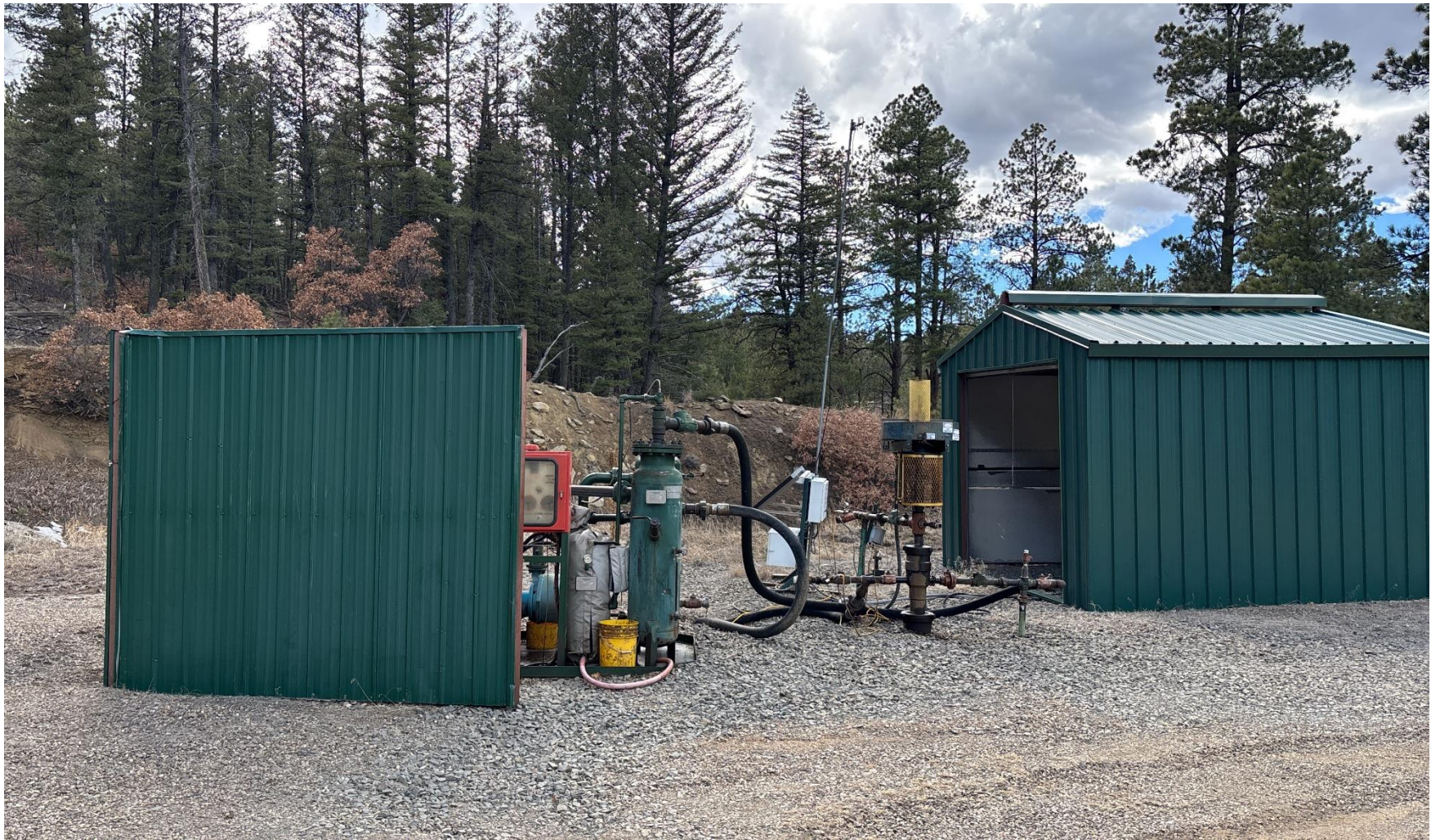
PHOTO 3: WELLHEAD AND EQUIPMENT.
