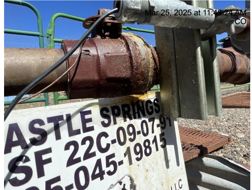
Photo # 6892 Mechanical Condition - Possible ball valve leak on CSF 22C-09-07-91 well
