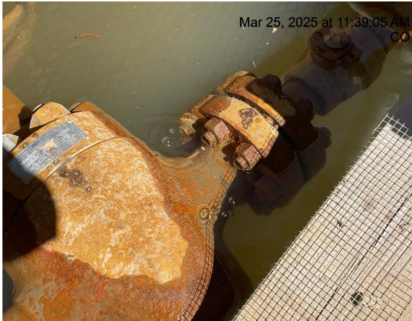
Photo # 6887 Mechanical Condition - Possible leak on CSF 44C-09-07-91 wellhead
