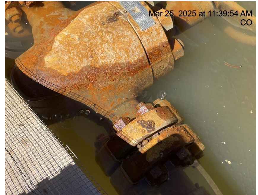
Photo # 6888 Mechanical Condition - Possible leak on CSF 44C-09-07-91 wellhead
