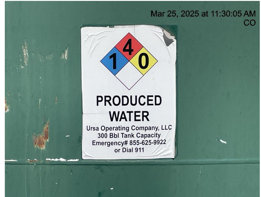
Photo # 6896 Tank label contains inaccurate information
