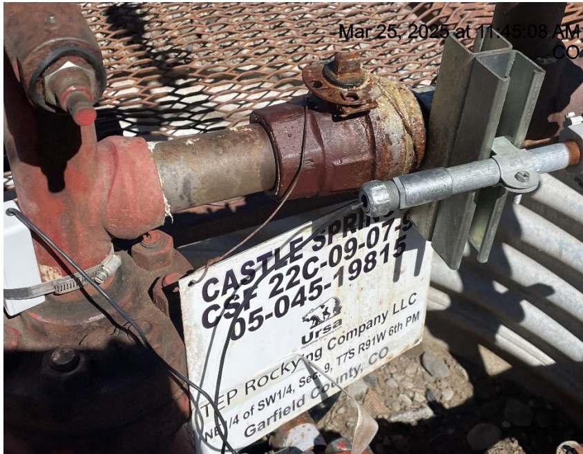
Photo # 6889 Mechanical Condition - Possible ball valve leak on CSF 22C-09-07-91 well
