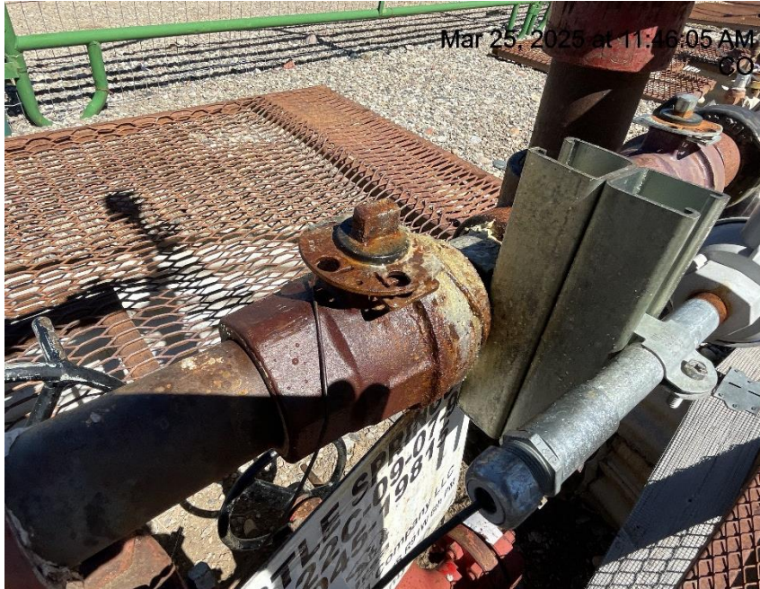
Photo # 6891 Mechanical Condition - Possible ball valve leak on CSF 22C-09-07-91 well
