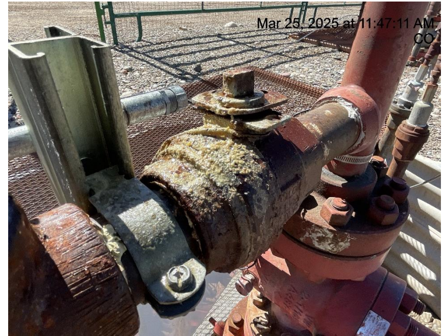
Photo # 6890 Mechanical Condition - Possible ball valve leak on CSF 22C-09-07-91 well
