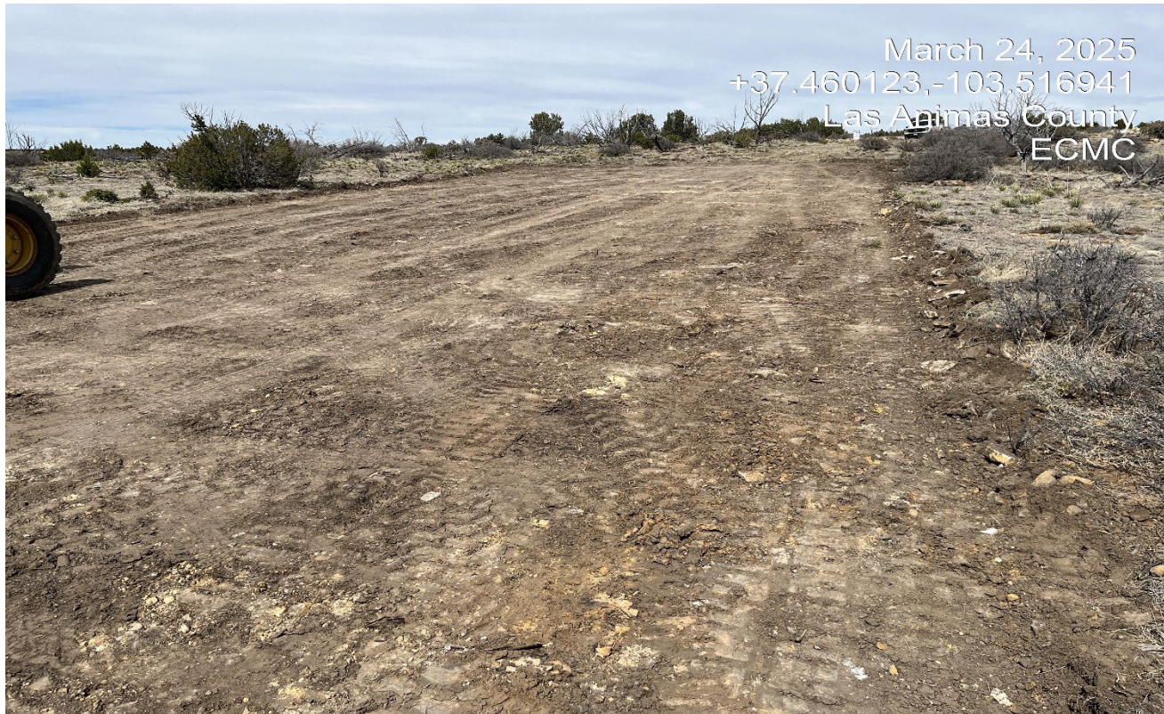
Photo 6. Facing northwest at the location. There were no stormwater BMP's installed at the location at the time of inspections. BMP's need to be installed prior to construction.
