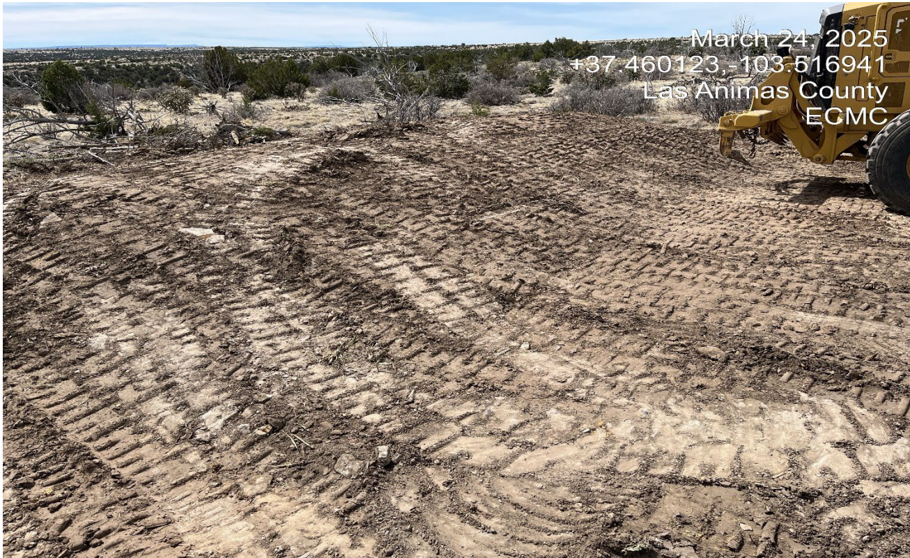
Photo 5. The topsoil pile has been stored at the south side of the location and was tracked for temporary stabilization..
