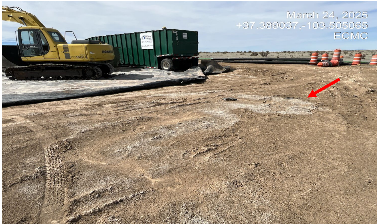
Photo 6. There are stained soils where fluids have leaked off the
