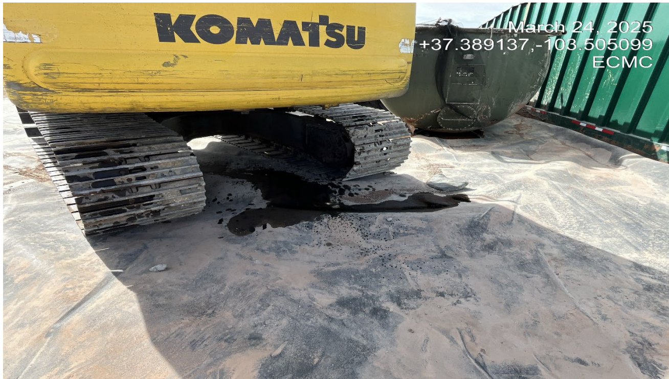
Photo 7. The excavator had a leak but was parked on the liner.
