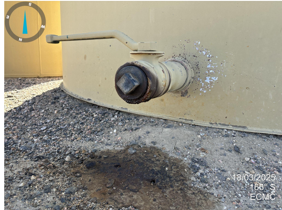
Photo 4. Stained soil and leaking valve at western tank.
