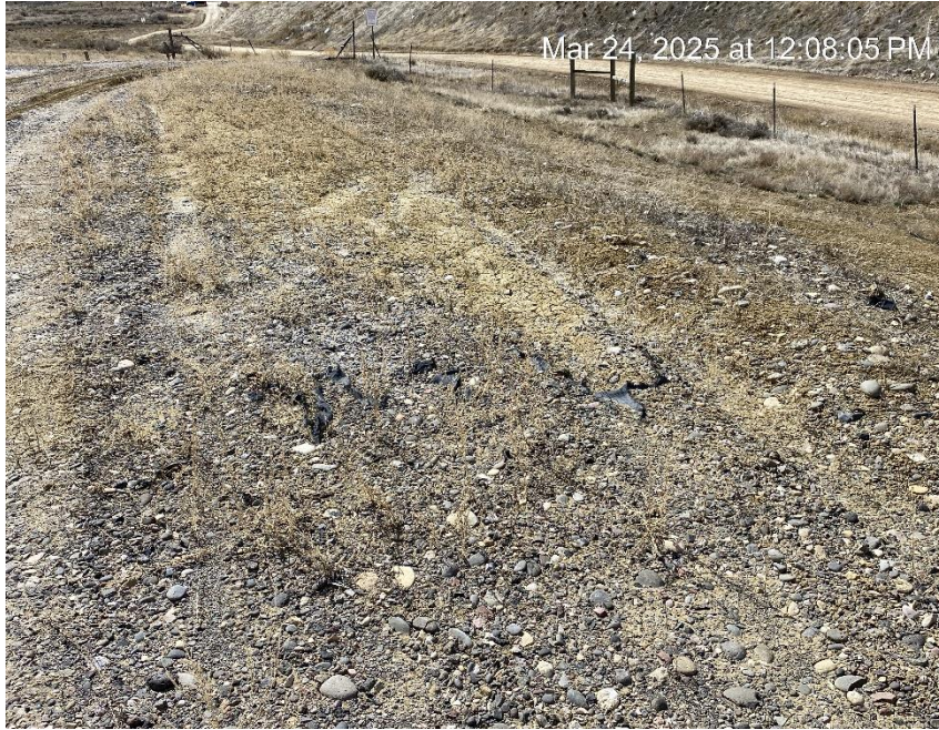
Erosion and sediment migration
