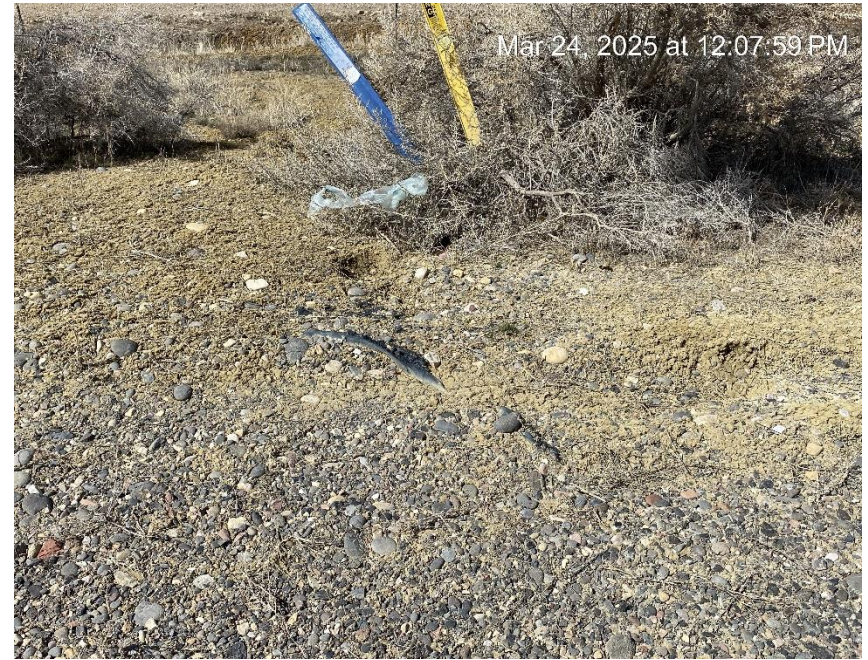
Erosion and sediment migration
