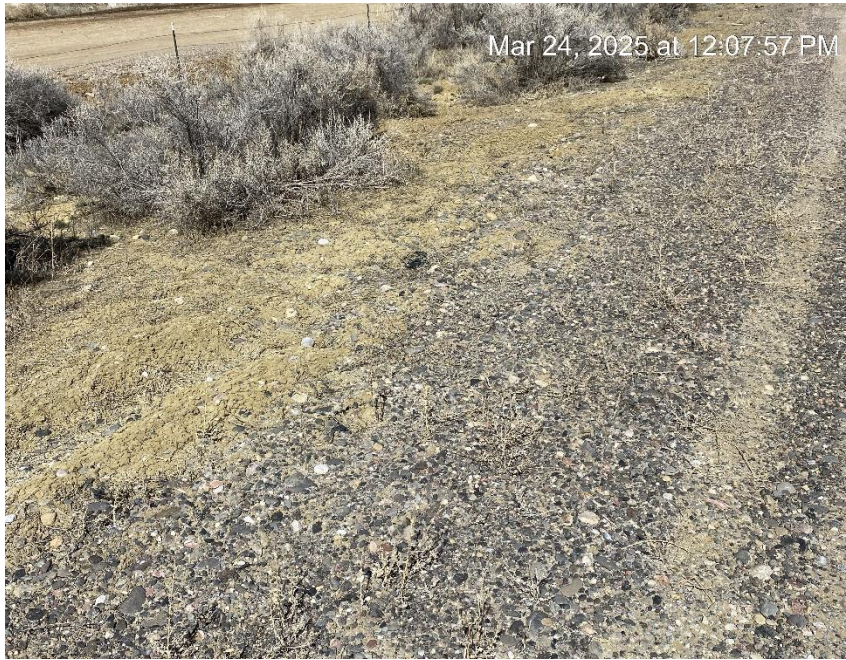
Erosion and sediment migration
