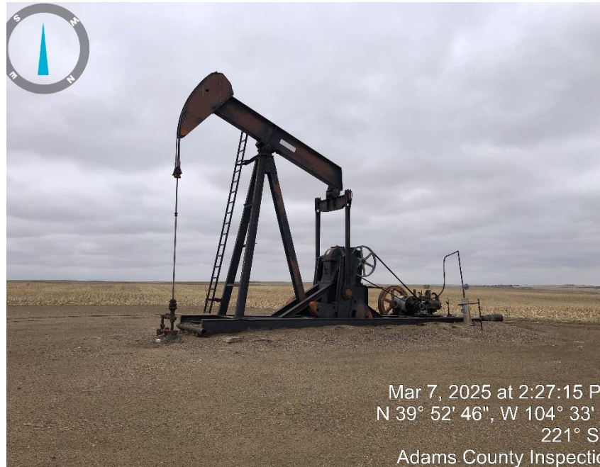
Photo #3 Pump jack.
