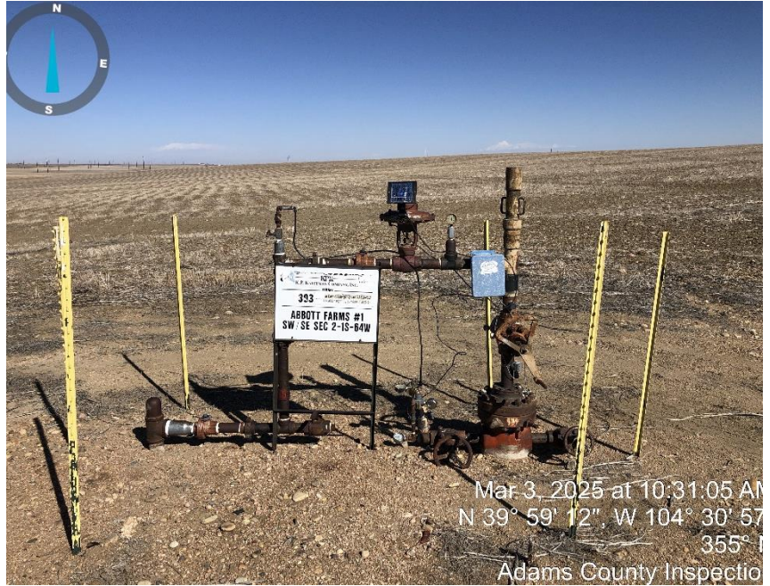
Photo #4 Well head.
