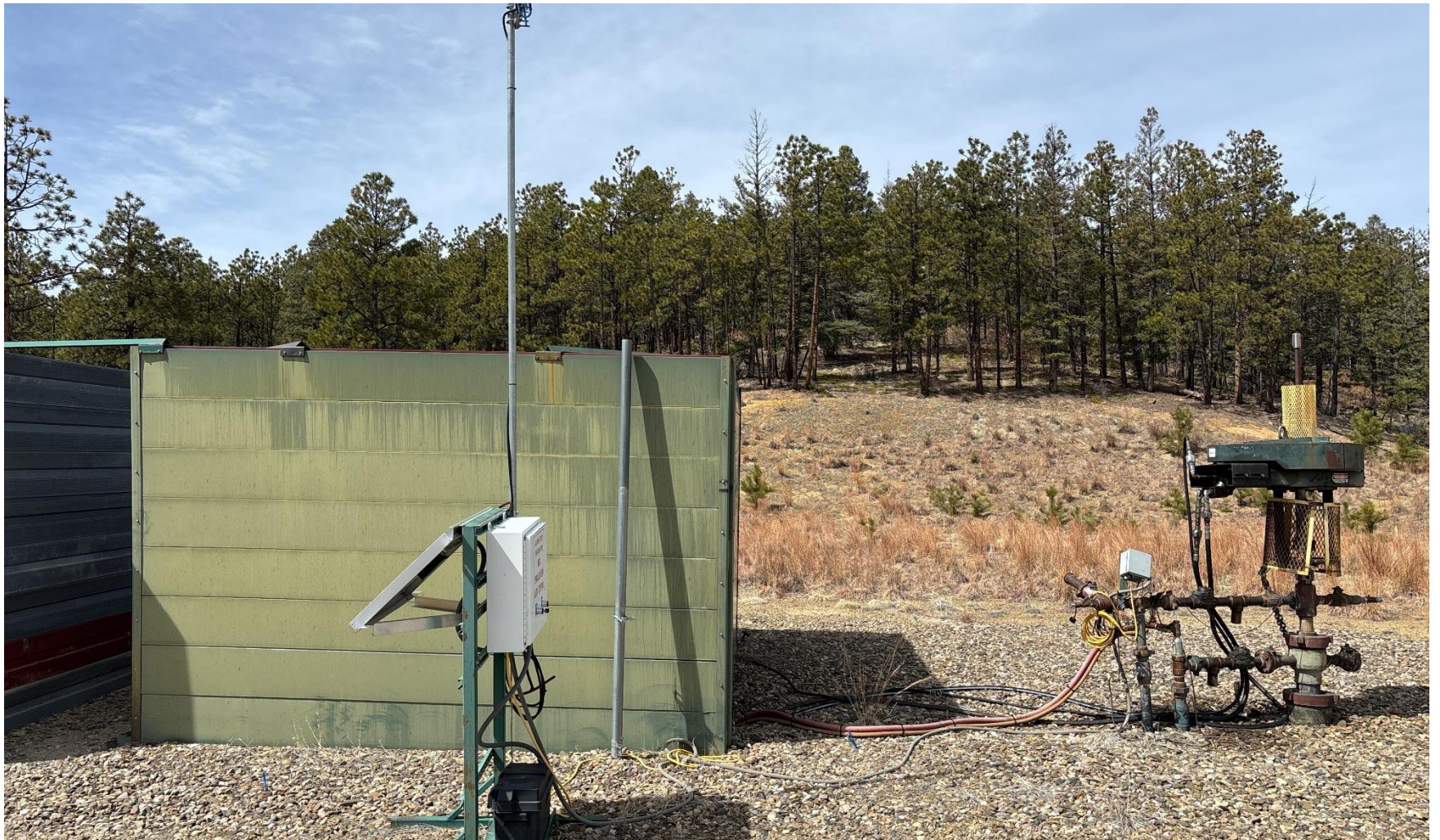
PHOTO 3: WELLHEAD AND EQUIPMENT.
