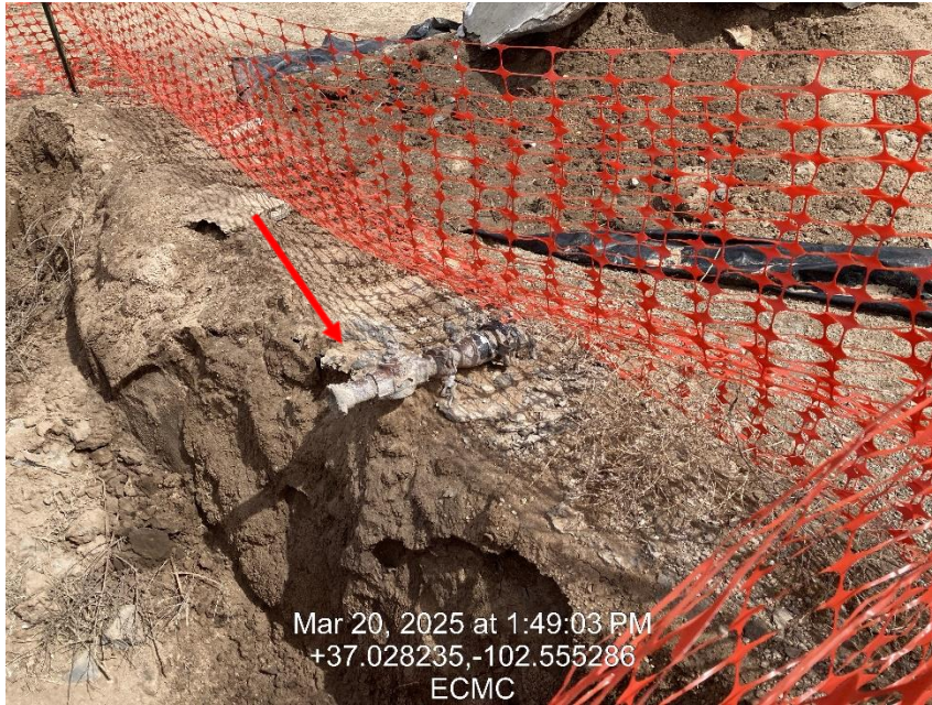
Photo 11 – Flowline at wellhead
