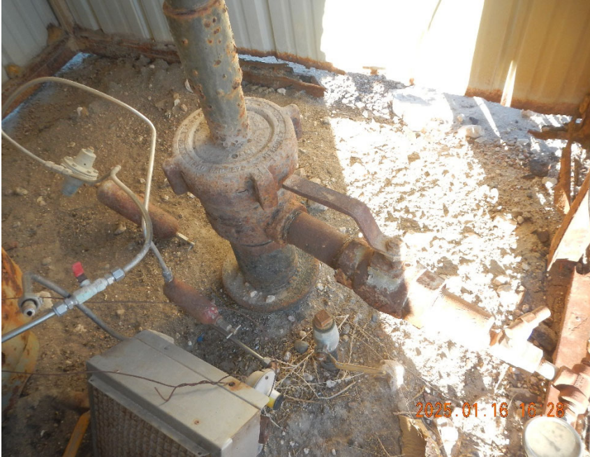
3. View of wellhead. Note debris on ground inside shed 01/16/2025.
