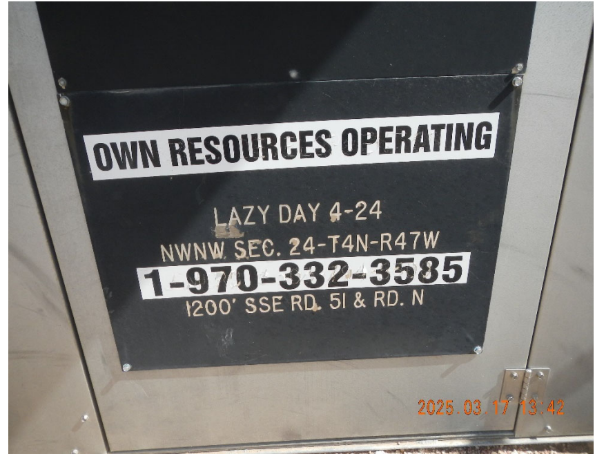
2. Lease sign at shared gas meter run on 03/17/2025.
