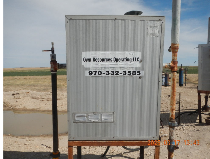
4. Separation equipment as seen on 03/17/2025. Operator and contact information added. No associated well information.
