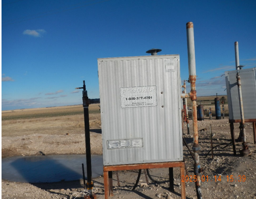
3. Separation equipment as seen on 01/14/2025.
